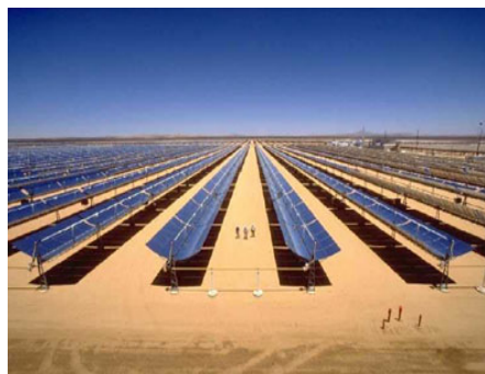
Parabolic trough solar thermal technology
